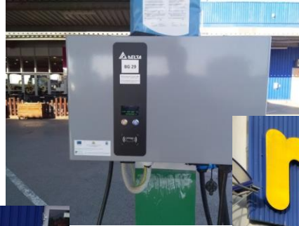
MCC Bulgaria, Sofia – Upgrade to DC charging
